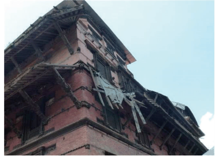
(a) 柯提普塔(Kirtipur Tower)斜撑坠落
