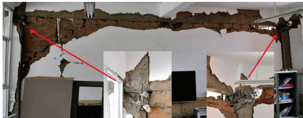
(e) ⑥轴横墙框架柱剪切破坏
